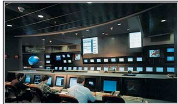
Fig 1: Command and Control center with many sources/displays
